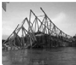
Kapuas Timpah Bridge April 3, 2009 Collapsed because of design flaws.
